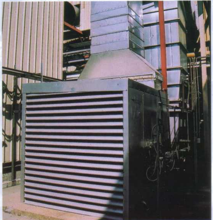
Recovered heat from the ABB dryers is recirculated through the pocket ventilator. Installation of the gas dryers reduced the need for a separate burner within the ventilator.
