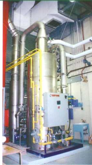
“Ultra-High Efficiency” direct contact water heater installed at the Neufchâtel Professional Formation Centre
