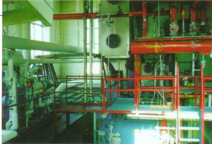
Dual temperature direct contact water heater installed at the Sorel General Hospital
