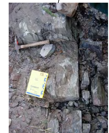
3 OPEN JOINTS, CALCITE FILLED SPACING : 0.05 TO 0.5m GREENISH MASSIVE BEDS OF MUDSTONE
