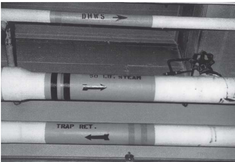
Controlled products in pipes identified by colour and letters.
