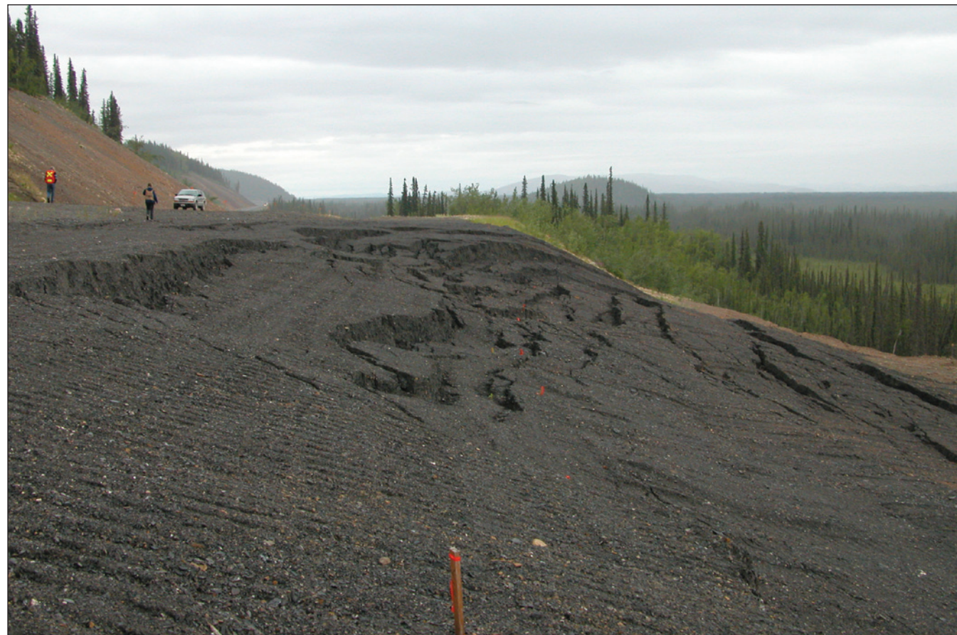
Subsidence of road fill along the Alaska Highway near Beaver Creek caused by permafrost thaw beneath fill. The failure is not directly linked to climate change — rather it was caused by disturbance of groundwater flow pathways which has led to permafrost thaw at this site. But it is representative of the type of failures that could occur along highways as permafrost starts to thaw more.
