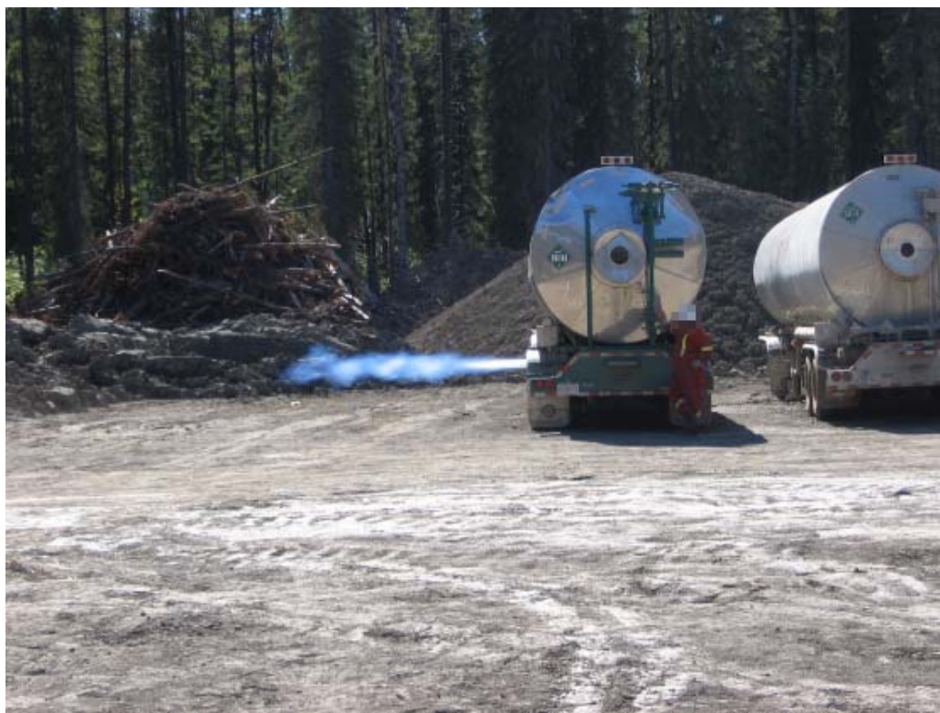
Photo 7: CO 2 is vented at a pressure of approximately 300 psi through a 4-inch-diameter pipe.
