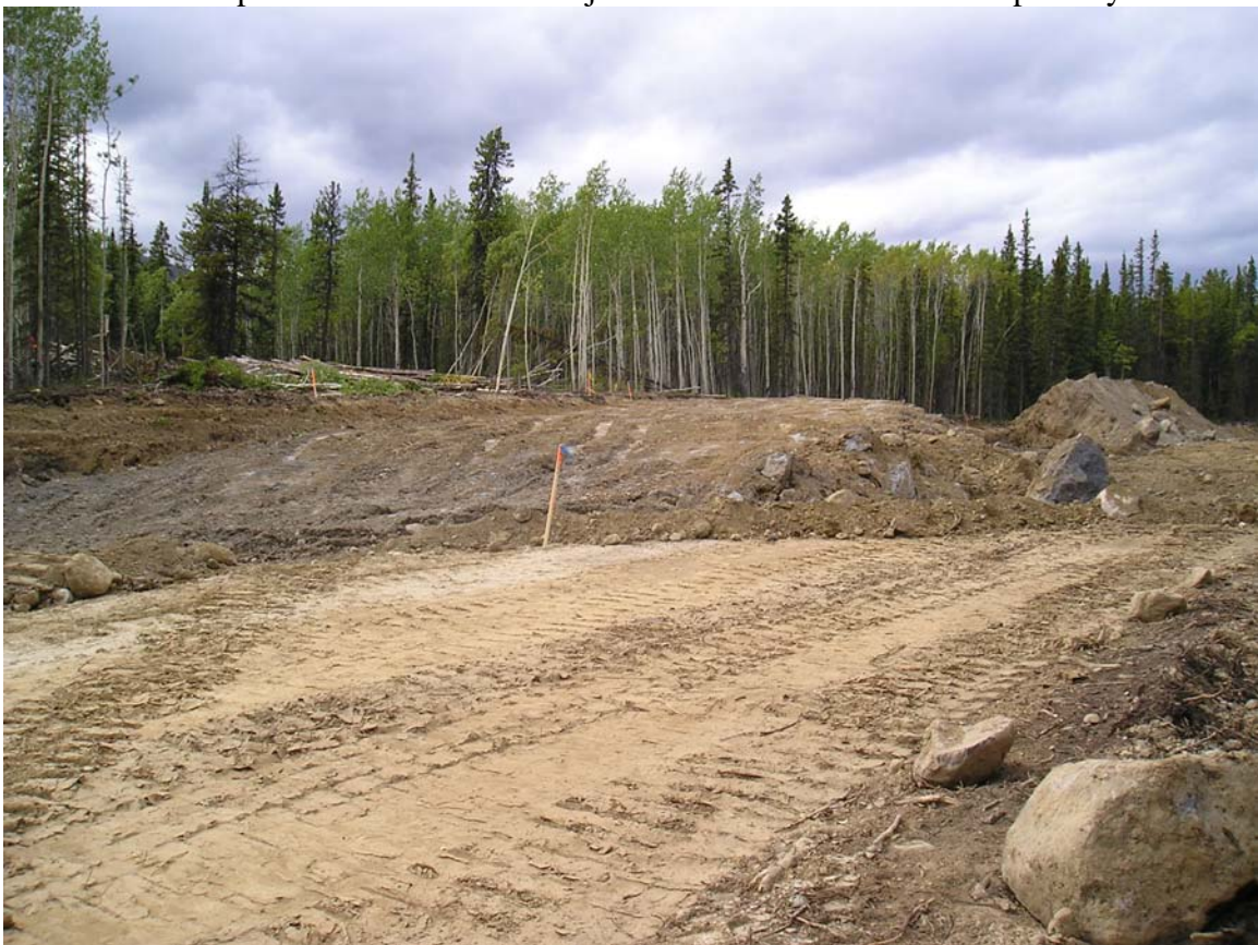
Rock Outcrop #3 on Collins Lane Adjacent to Lot 40 Prior to Blasting – August 2006
