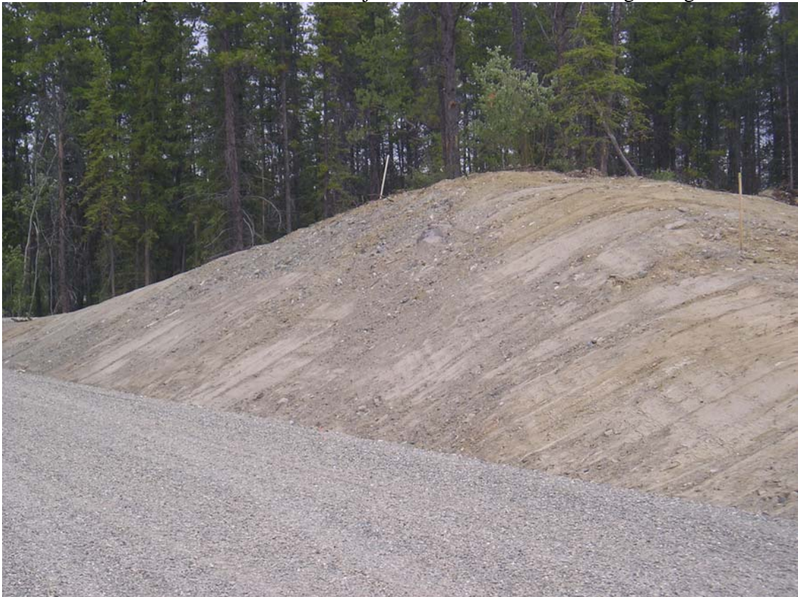
Rock Outcrop #1 on Levich Drive Adjacent to Lot 18 After Clean Up - July 2007
