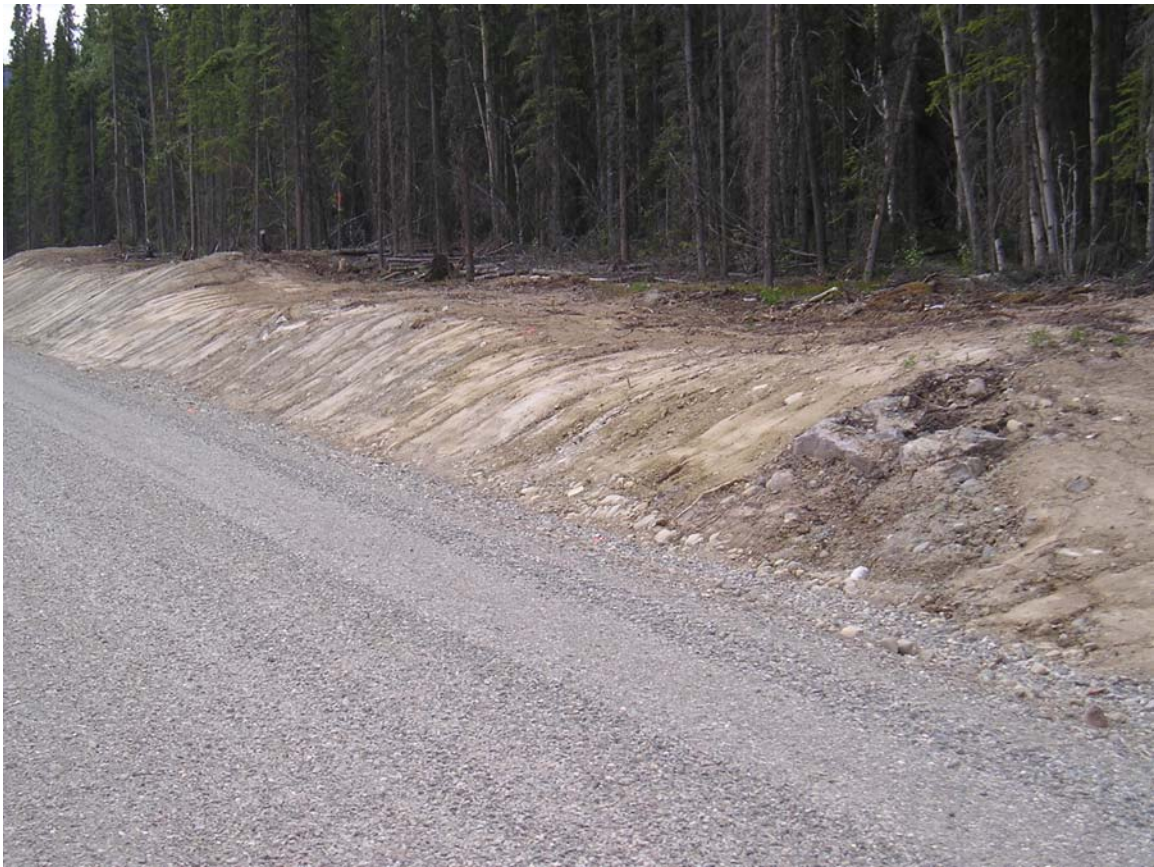
Rock Outcrop #2 on Levich Drive Adjacent to Lot 33 After Clean Up – July 2007
