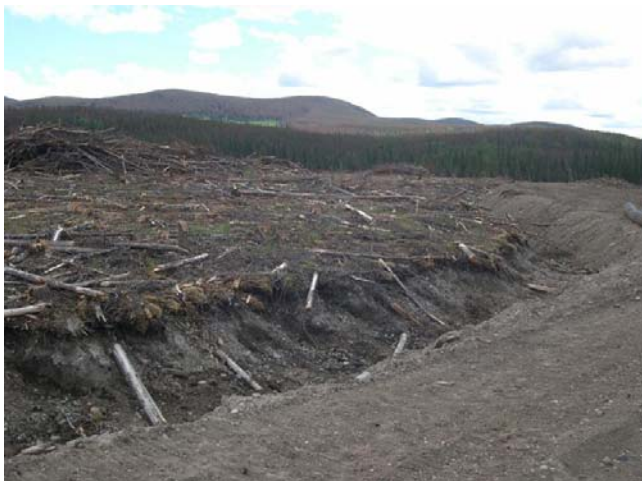
Figure 8: Roadside residuals may be situated across a ditch and away from the road.
