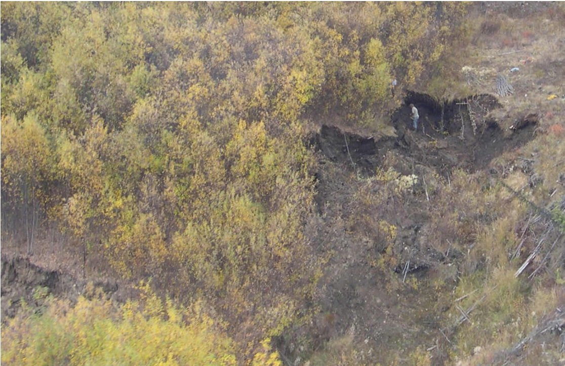
Aerial view of the upper portion of the cut. The completed structures on the east wall can be seen in the upper right. Stabilized section in the foreground. September 7, 2005.
