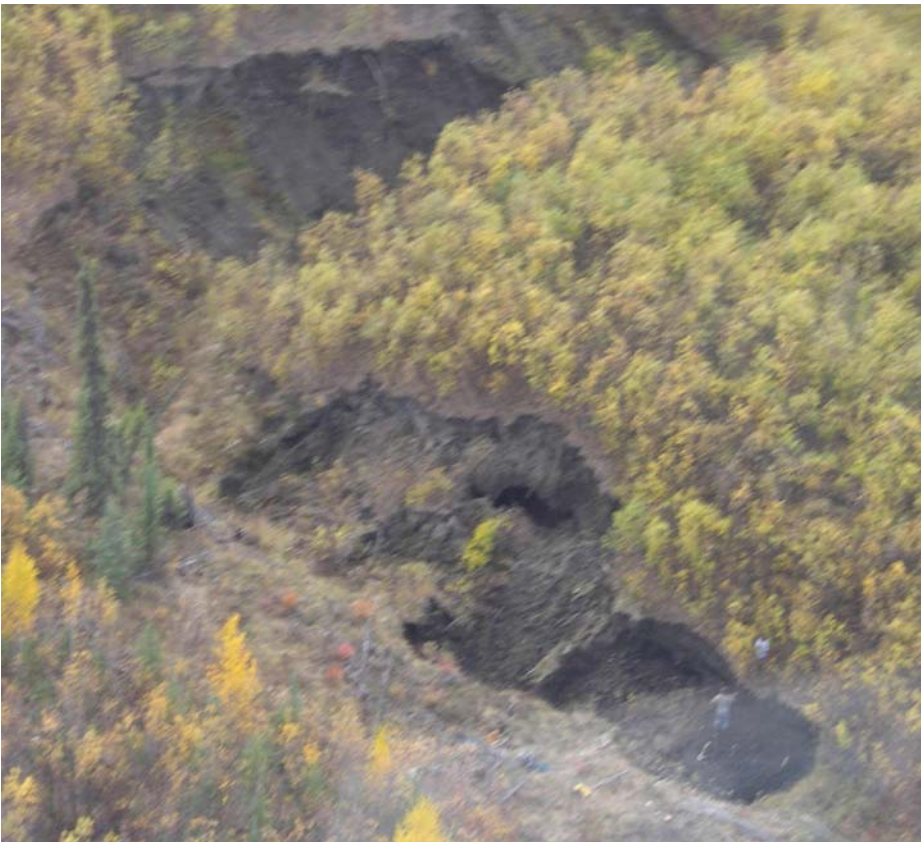
Aerial view looking back along the cut. Work is commencing on the west wall. Sept. 7/05
