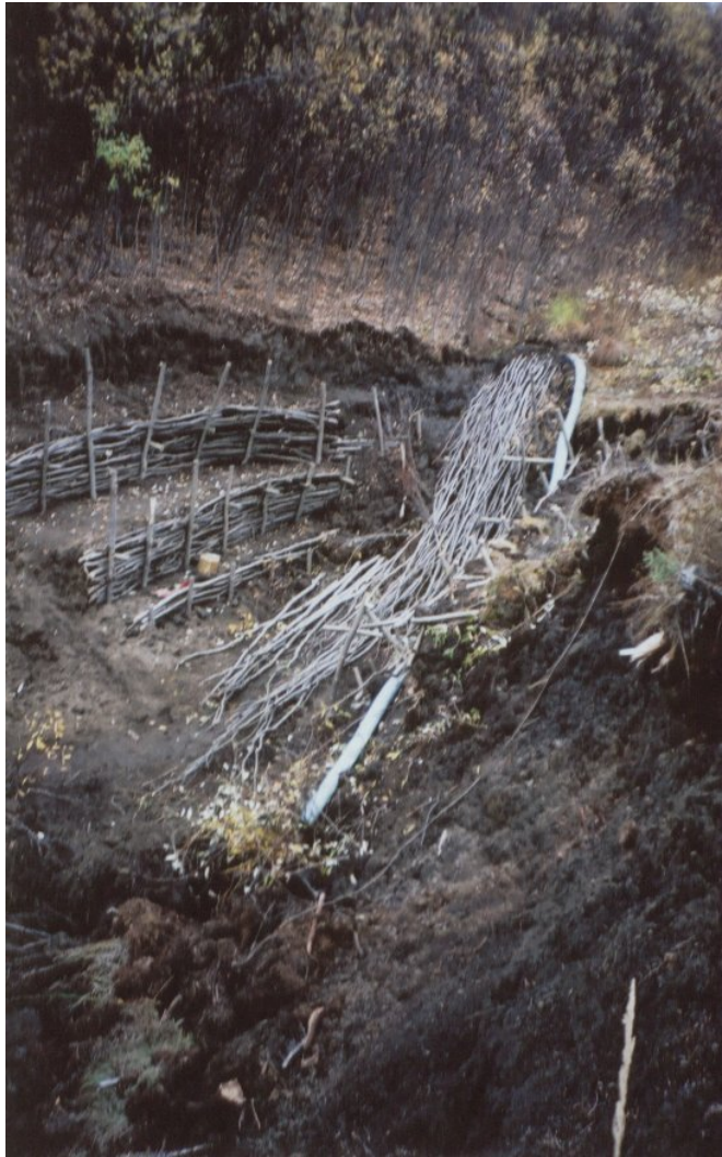
Live willow flume prior to the placement of cross willows. pipes installed. September 9 th , 2005.
