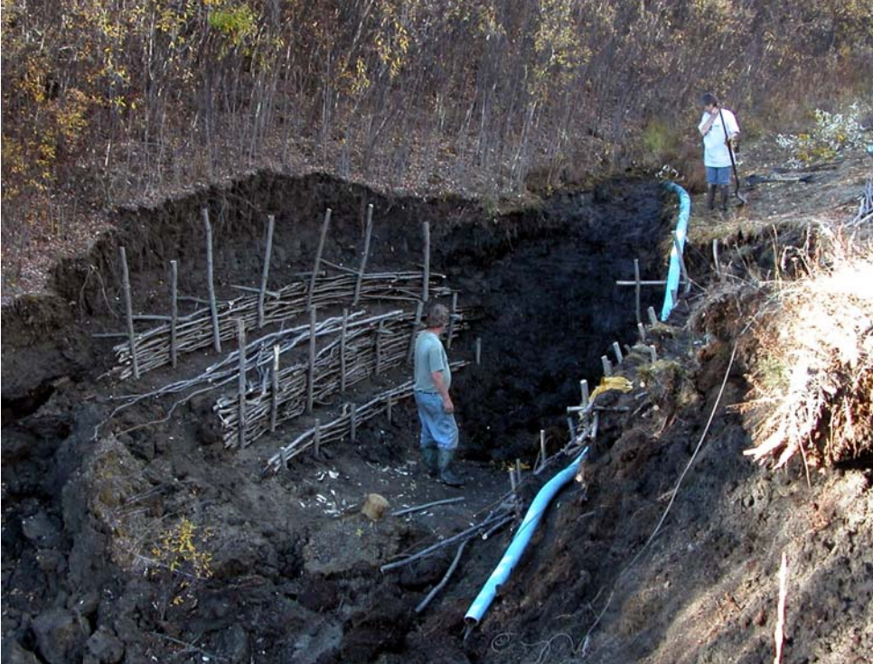
The two tiers of retaining walls have been backfilled in readiness for the installation of the live willow flume. September 9 th , 2005.
