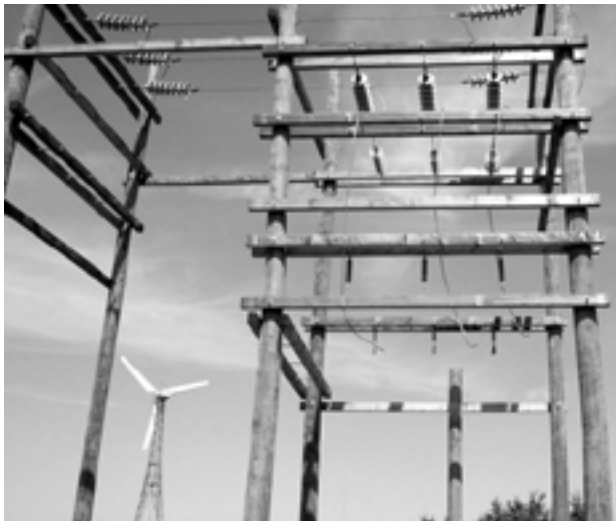
Wind power currently provides five per cent of PEI's electricity. Above, the North Cape substation frames one of the turbines at the Atlantic Wind Test Site.
