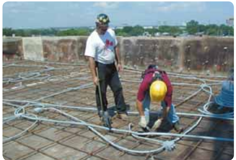
The Research Advisory Council invites projects to study better safety practices. One of the dozens of successful projects in 2004 was the automatic rebar tying machine , which decreases forceful hand exertion, repetitive hand motion and improves ergonomics.
