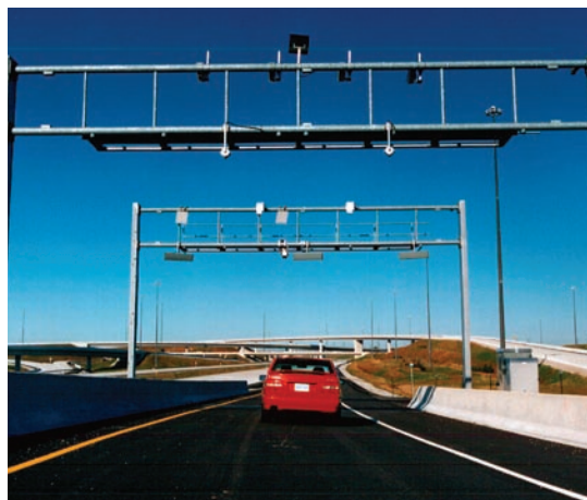
Electronic tolling system automatically bills users or charges their account without the need to slow down or handle change.
