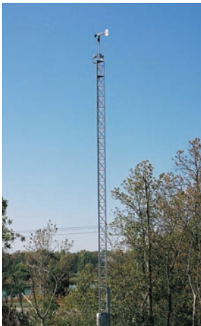
Advanced Road Weather Information System (ARWIS) monitor and detect weather and road conditions.
