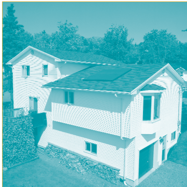
▲ Glazed flat plate collectors installed on a Nova Scotia home.
