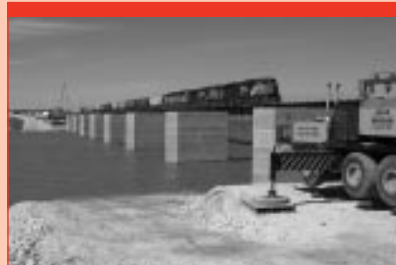
Installation of the temporary bridge piers at the Sprague Railway Bridge was temporarily suspended when the floodway was operated in the spring of 2006. During the spring, the floodway prevented over $2 billion in flood damages in Winnipeg.
