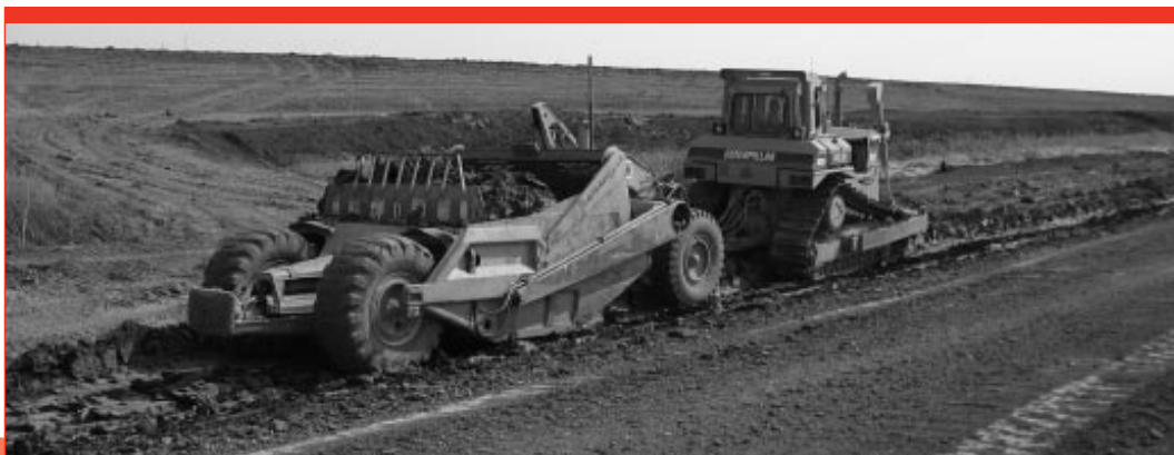
Work on part of the West Dike has been awarded as part of the Aboriginal Set-Aside.
