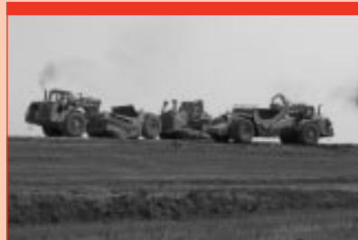
Work on the West Dike will improve protection against wave and wind action during major flood events.
