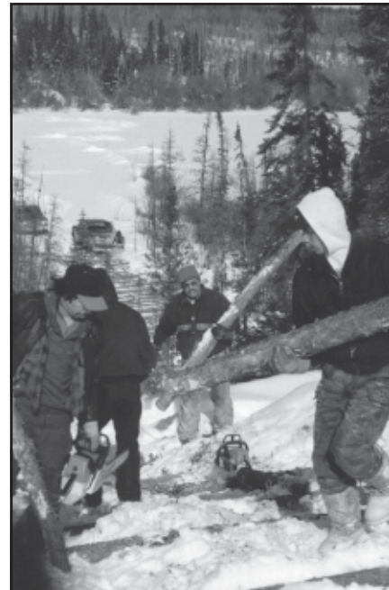
Split Lake project workers installing bank stabilization works at the crossing of the Pukatawakan River, in keeping with the requirements of the Environmental Protection Plan for the project.
