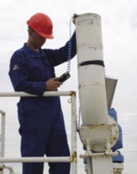
Screening for fugitive emissions at a natural gas pressure regulating station
