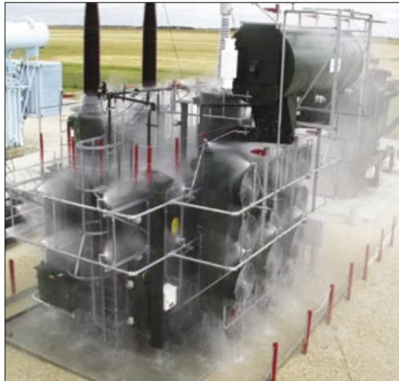
Testing a fire protection system that showers water over an HVDC converter transformer at Dorsey Converter Station
