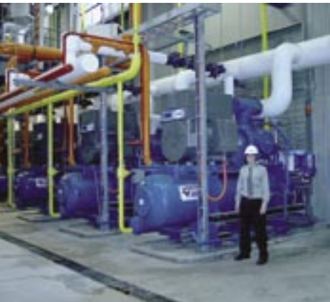
Compressors in "refrigeration alley" at Simplot. They are capable of freezing more than one million pounds of french fries a day as well as other potato products, and keeping buildings cool.
