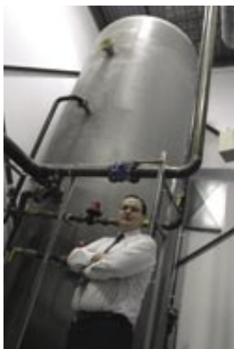
One of two, 2-storey-high 10 000-gallon air storage tanks for the engine test air system. The tanks are one of the keys to an energy efficient compressed air system for Standard Aero.
