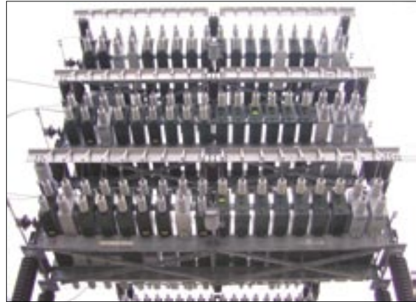
Banks of capacitors containing PCBs, at Dorsey Converter Station. These capacitors will be replaced with PCB-free versions.
