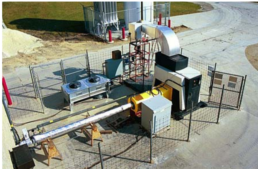
Microturbine installation for demonstrating odour control at Winnipeg's South End Water Pollution Control Centre.
