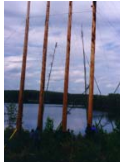
Woodpecker holes appeared in a pole at a river crossing of the North Central transmission lines — only two years after installation. The lower nest-hole could threaten the structural integrity of the pole because of its position so close to the attachment point of the guy wires.
