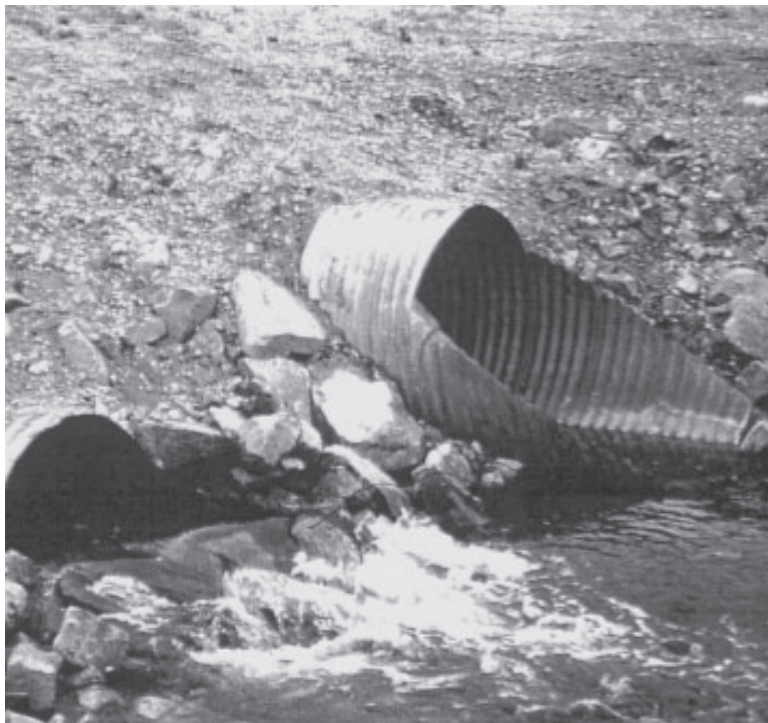
Culverts installed at different elevation in Sundance Creek to enable fish passage at high and low flows.
