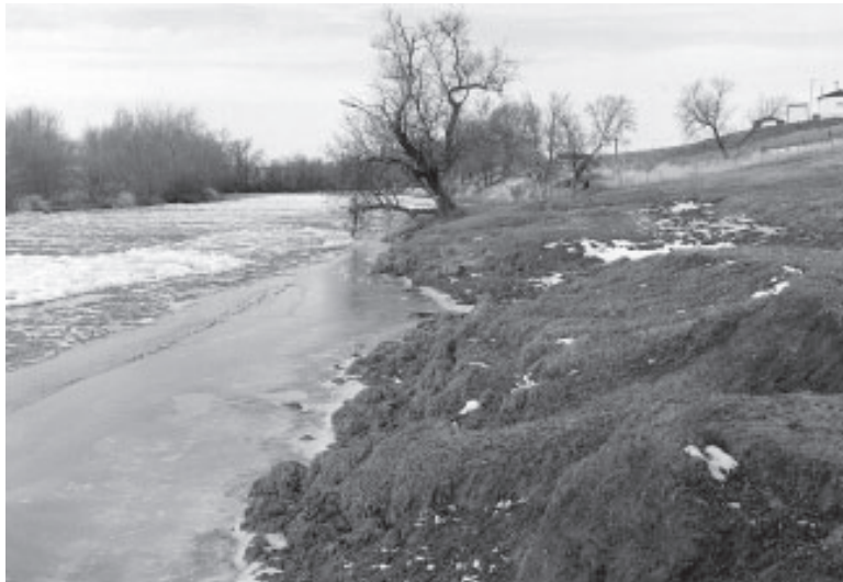
Erosion and sedimentation result from removal of stream bank vegetation.
