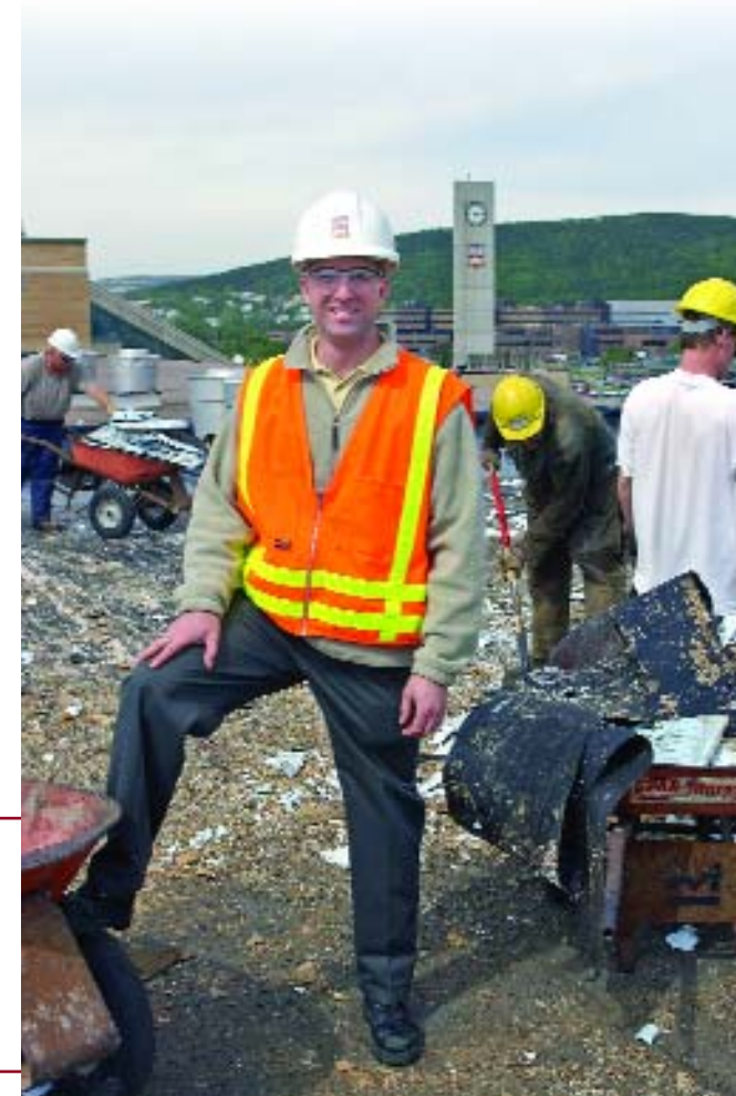
Boyd Ash, project technologist with Facilities Management, on the roof of the Science Building on Memorial's St. John's campus. Annual roofing repairs are well underway again this year.
