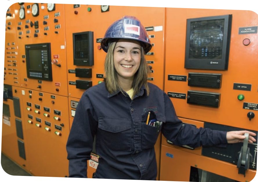
CRYSTAL BUTLER IS IN CONTROL OF HER FUTURE CAREER CHOICE AS AN INDUSTRIAL ELECTRICIAN.
