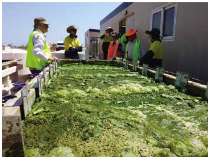
Muradel's unique algae harvesting system at the Karratha Pilot Plant
