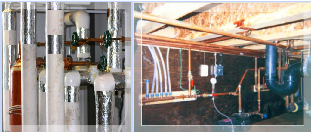
Northern plumbing examples
