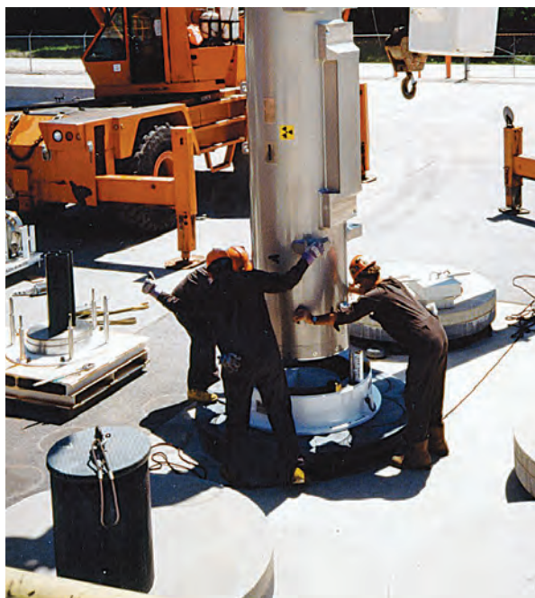
Intermediate level waste is inserted into an in-ground storage container at the WWMF.
