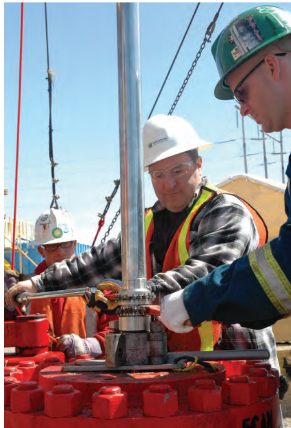
Westbay groundwater monitoring equipment provides data to ensure groundwater quality isn't compromised.
