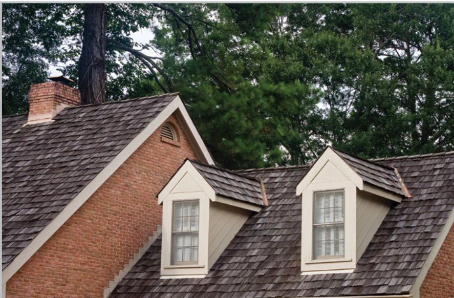
Figure 10 Roofing material, such as wood shingles, can impact the quantity and quality of rainwater you can collect
