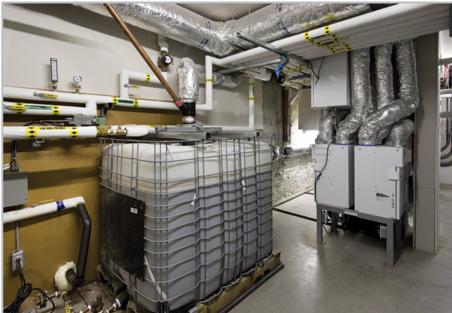
Figure 8 This 1,000-L indoor rainwater tank, which supplies water for toilet flushing in three apartment-style condominium units, is equipped with a top-up system to ensure water is always available
