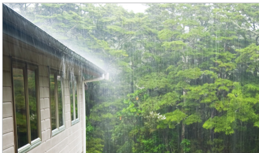
Figure 11 Overflowing eavestroughs that are free of debris can indicate improperly-sized or sloped eavestroughs or an incorrect number of downspouts to drain the eavestroughs
