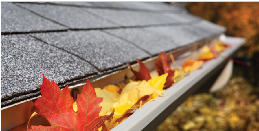
Figure 26 To keep your system in good working order, it is important to regularly trim back overhanging trees and prevent debris from accumulating in eavestroughs and downspouts
