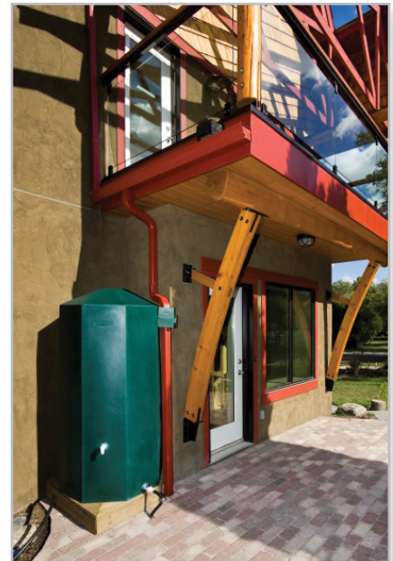
Figure 2 Rainwater harvesting at its simplest: a rain barrel placed below a downspout
