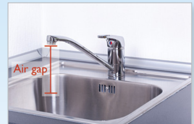
Figure 18 An air gap prevents drain water from backing into, and contaminating, the potable water supply from the tap
