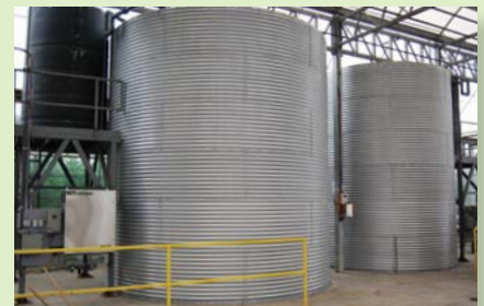
Store clean water in durable, waterproof storage tanks.
