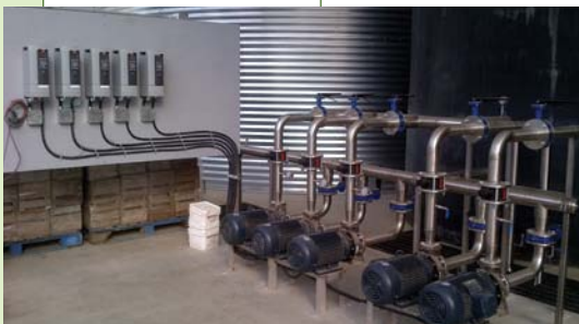
Use of technologies such as variable-speed soft-start irrigation pumps improves precision of irrigation scheduling.
