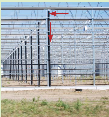
This greenhouse under construction features downspouts to direct rainwater to storm water retention pond.
