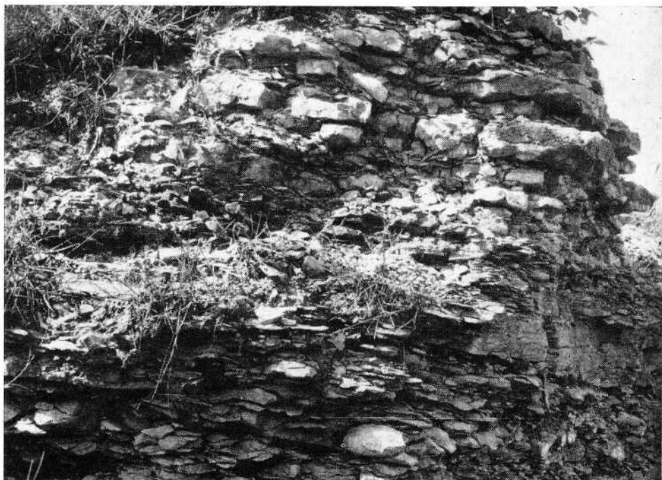
This picture shows the friable nature of the underlying limestone bedrock. The limestone is seamed and interbedded with shale partings.
