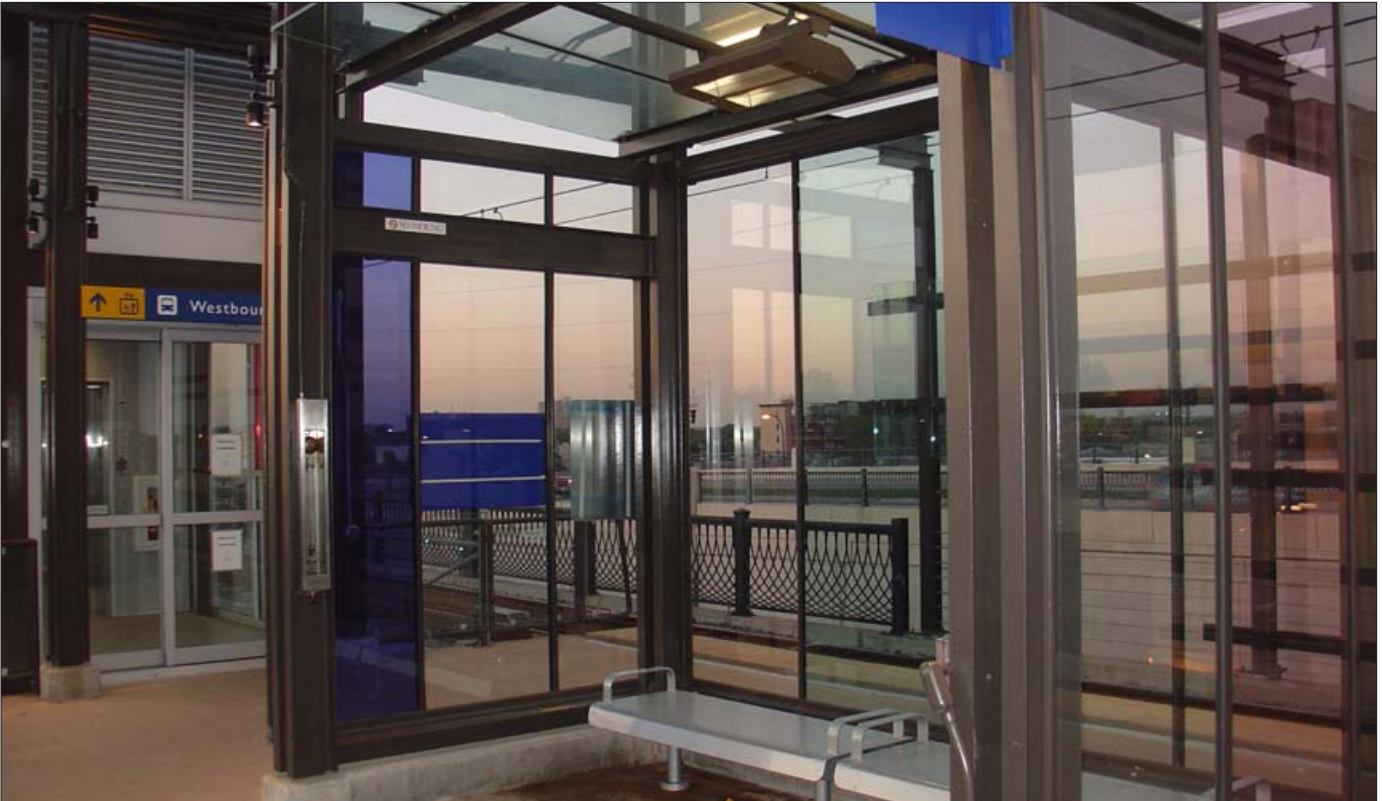
A shelter within a transit station in Saint Paul MN, incorporates user-activated radiant heating in order to enhance passenger comfort during colder winter months.
