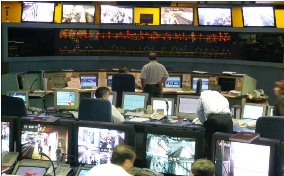
An asset management plan can account for the lifecycle costs of a range of physical assets such as computers or control systems that are critical to the operation of the transit system.
