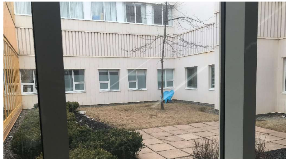
Picture: Queen Elizabeth Hospital - Unit 9 and 9A Client Recreation Space, QEH Courtyard Source: Queen Elizabeth Hospital Facility Tour, March 2018
