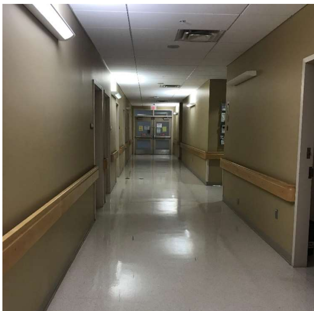
Picture: Prince County Hospital – MH Unit Hallway Source: Prince County Hospital Facility Tour, March 2018
