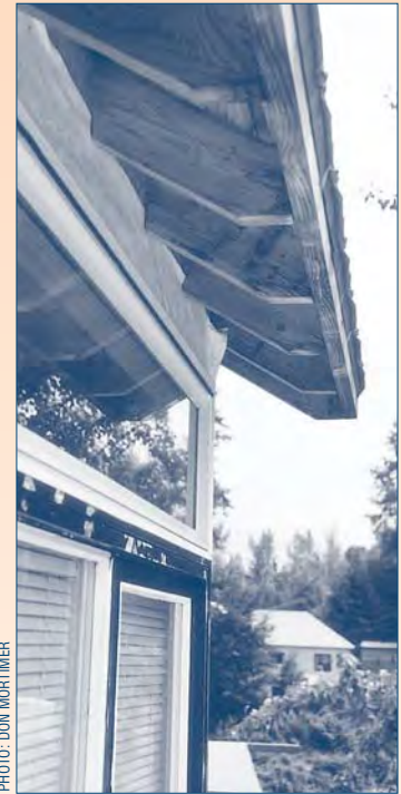
▲ Open eaves, vents not screened. (6 pts)
